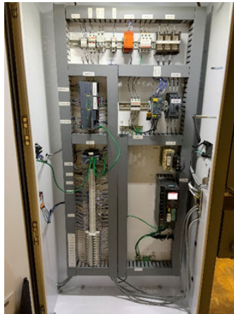
Figure 6: Typical PLC Control Cabinet
